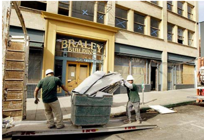
Construction materials are taken out of the Braley Building as a part of a renovation by the Church of Scientology in Pasadena Friday January 8, 2009. (SGVN/Staff photos by Walt Mancini)
