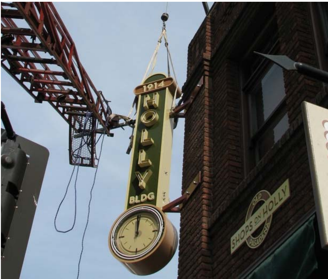
A view of the brand new "antique" clock after it was hoisted into position.
